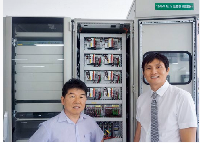
Key Yo, Managing Director of Tri-TEK (left) and Lee In-Eung, Managing Director of the Power21 Corporation, in front of a control cabinet
